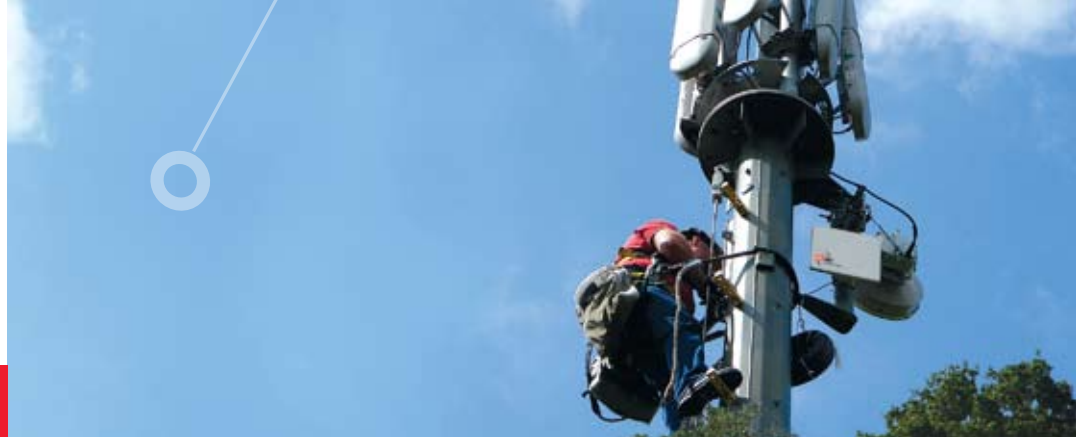
Cellular backhaul installation, USA
