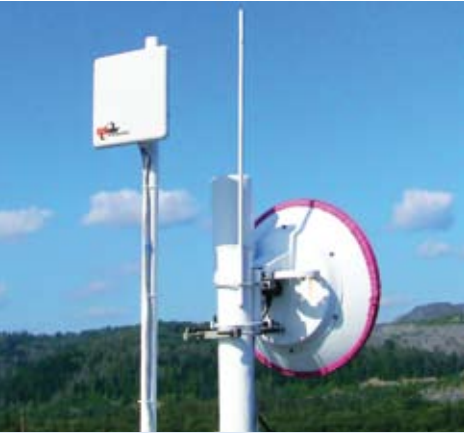
Gas utility connectivity, Siberia
